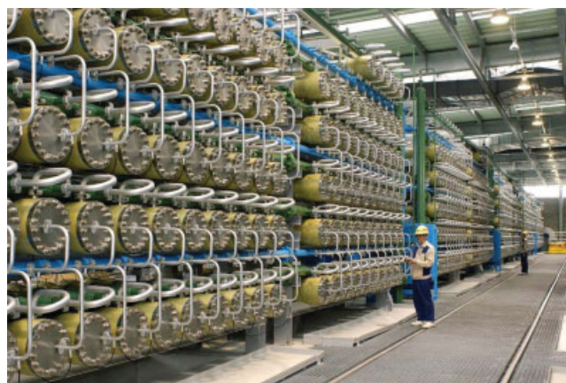
Figure 14 Photo of seawater RO modules for high recovery system in Fukuoka desalination plant in Japan (50,000 m 3 /d). [Color figure can be viewed in the online issue, which is available at www.interscience.wiley.com .]
